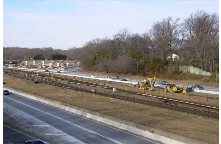
Pier guideway construction underway at the I-66 and Dulles Connector Road (Route 267) interchange. Photo by Dulles Corridor Metrorail Project
