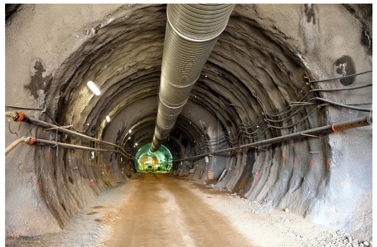
The outbound tunnel that will carry rail between Route 123 and Route 7 in Tysons Corner is currently more than 500 feet long and passes completely under International Drive. Photo by Rich Silva, Dulles Corridor Metrorail Project
