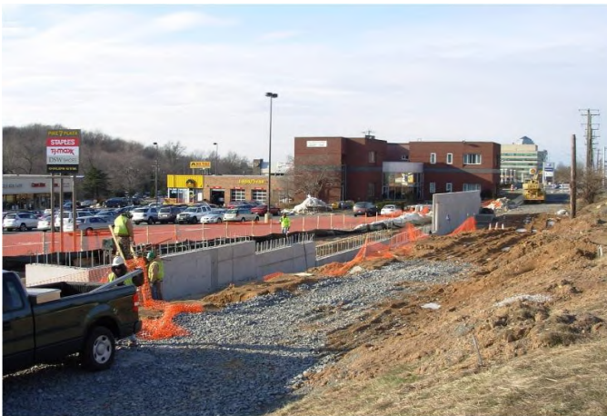
Construction of retaining walls on Route 7, necessary to build up the service roads to the same grade as Route 7 for lane shifting. Photo by Dulles Corridor Metrorail Project
