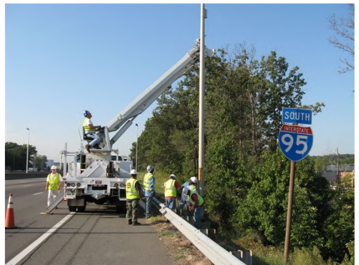
Virginia Department of Transportation 4 th Lane Widening Project; Portico is installing the electrical lighting & sign structures for Shirley Contracting.
