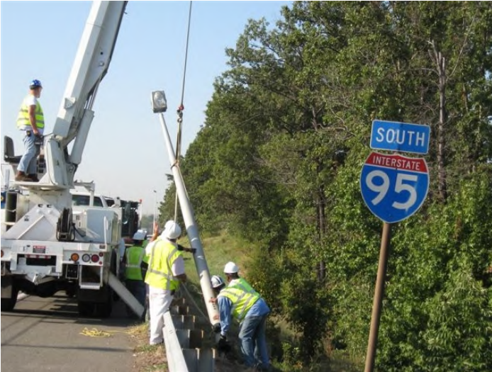
Construction began in March 2008 to add a fourth lane in each direction on I-95 between the Fairfax County Parkway and Route 123.
