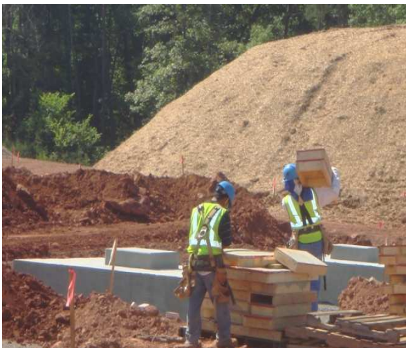
NIS workers perform foundation construction at the Dulles Corridor Metrorail Project pre-cast plant
